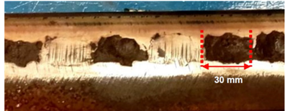
Typical spalling, Koekange (Dekra Rail, 2016)
